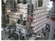
Electrical Heat Tracing System on EPCC Basis
